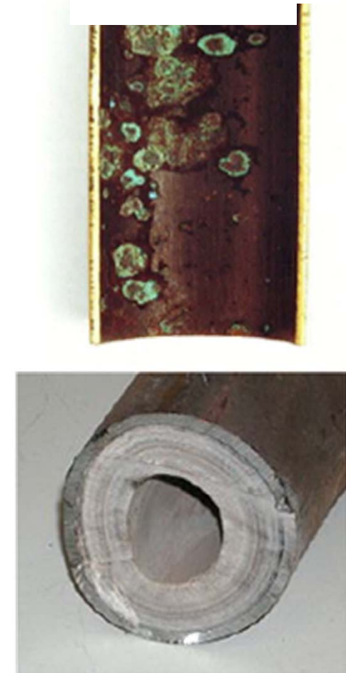
Water Side Fouling
