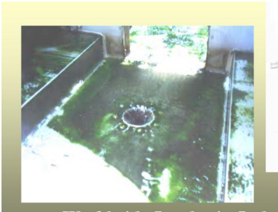
Algae formation in crossflow cooling tower basin
